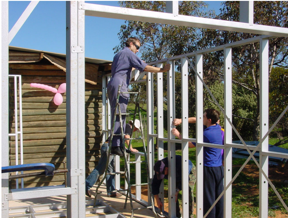
The clubhouse extension frames being 'erected' by Redmond and crew: Photo by D Conway
