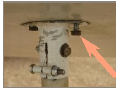
When DI'ing the MotorFalke always check that the bolts holding the wing walker legs on are tight and secure!
