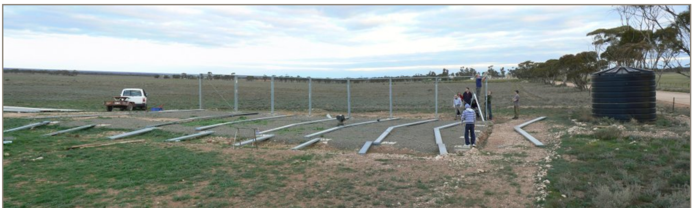
And then before anyone had realised it, Redmond had erected the southern wall of the hangar...
